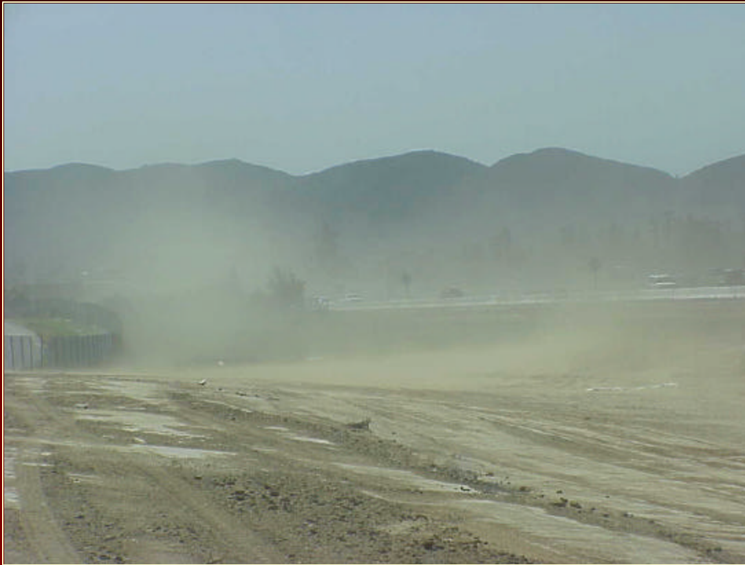
Lack of wind erosion controls
